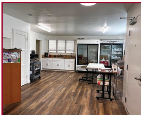
The renovation included a full makeover of the pantry area to allow for improvement in the daily emergency food distribution.
